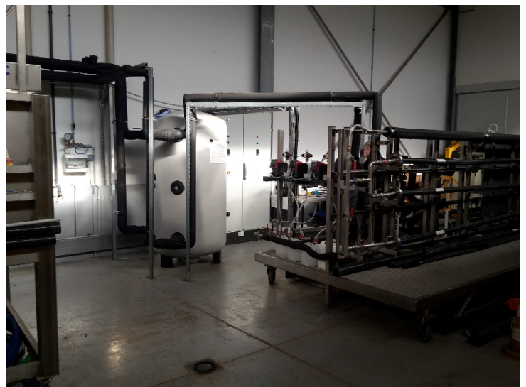
Figure 1: Installation pilote CVM
